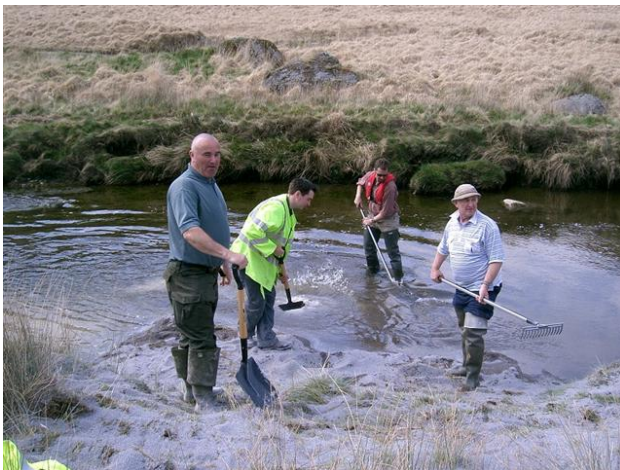
CRT and EAW staff getting "stuck in" to the delivery of limestone sand in 08/09.
