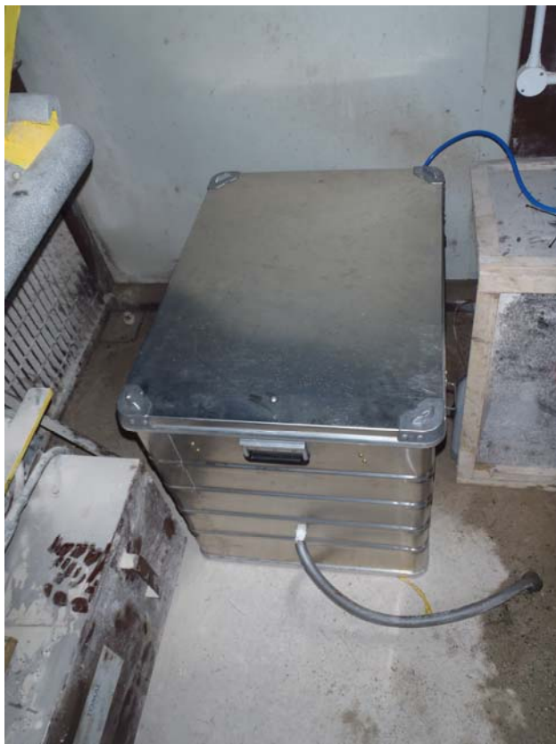
Fig 2. Unit housing the methanol generator which is being trialled at the Tywi doser. The generator operates automatically when required, to prevent the voltage falling below a level sufficient to operate the doser minimising downtime.
